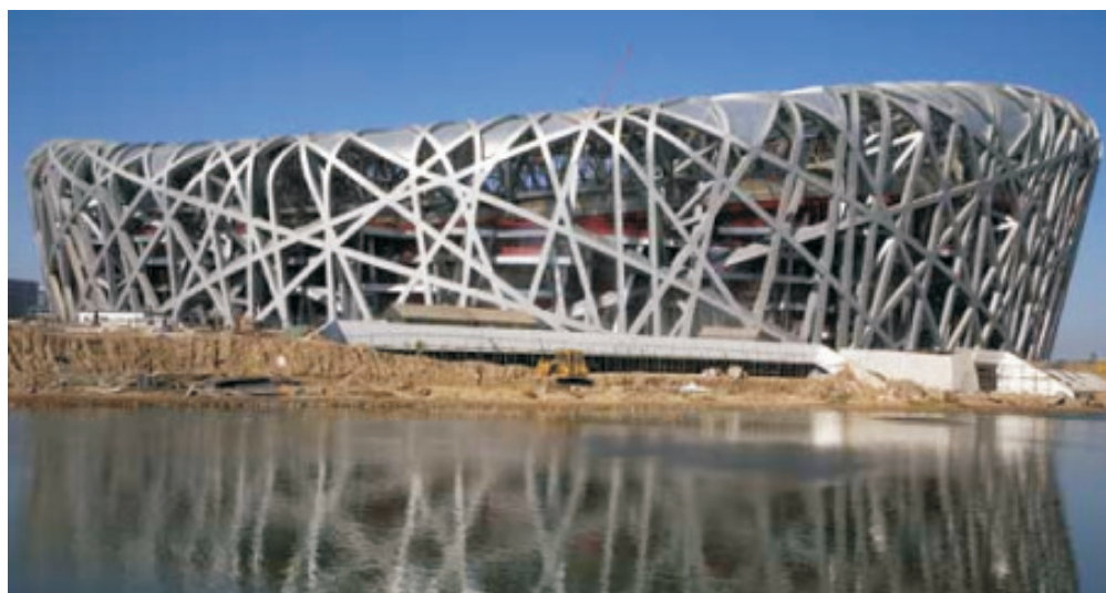
Figure1: The Beijing National Stadium (Bird's Nest), underconstruction (note the outermost layer of ETFE cladding at top) (source: Ref.4)
